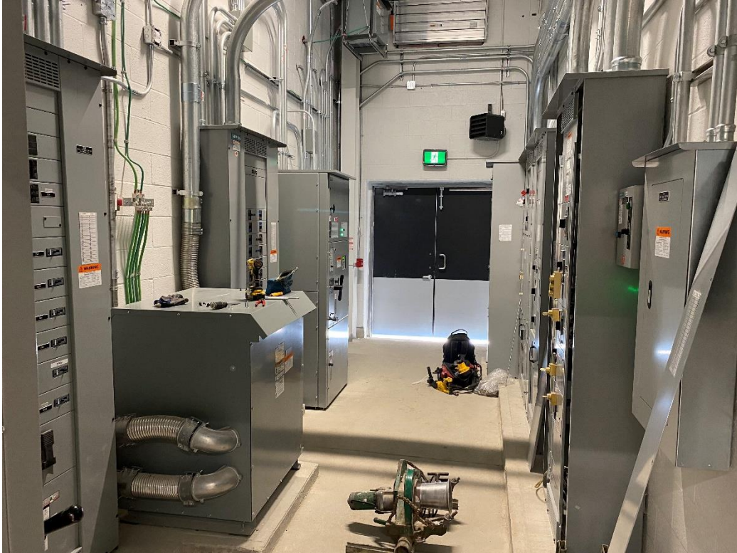
Main electrical room and switchgear
