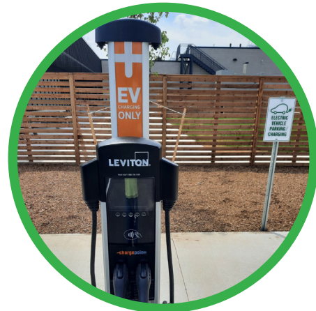
EV CHARGING STATION
