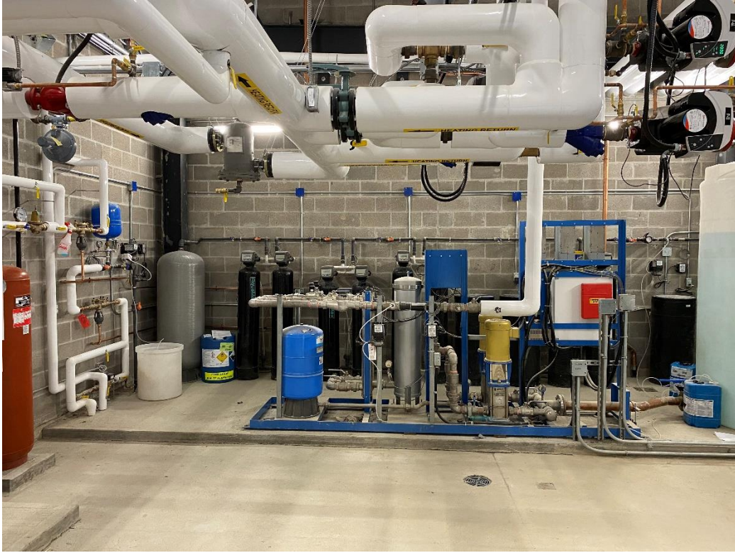
Mechanical room with water treatment system
