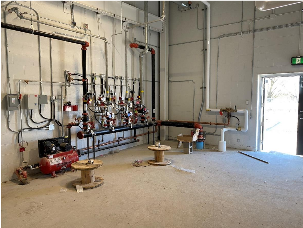
Sprinkler and fire suppression room
