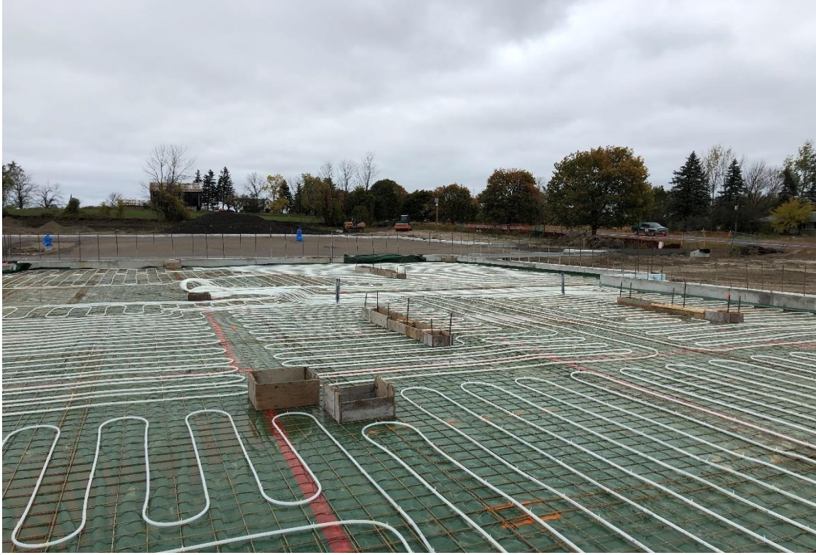
Underfloor heating along north elevation of administration area
