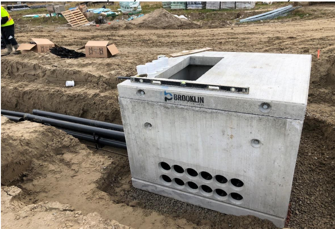
Transformer pad connecting primary and secondary duct banks
