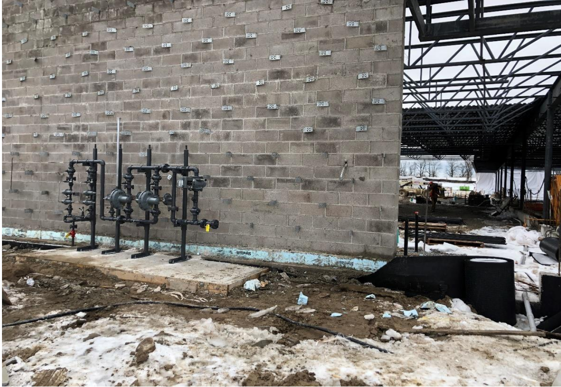
Enbridge Gas distribution station pad mounted along southern masonry wall
