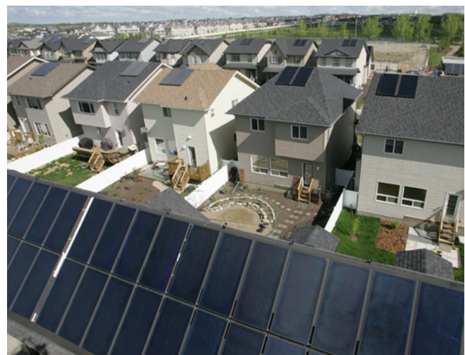
Solar panels on the roof of low-rise development.
